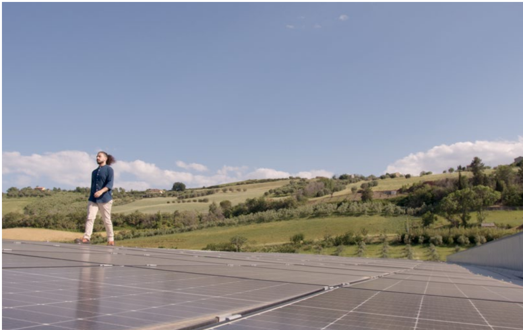
The photovoltaic plant at the Casoli di Atri (TE) location.
